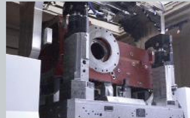
Direct loading of fixture on tilting/rotary table by means of 6-axis robot
